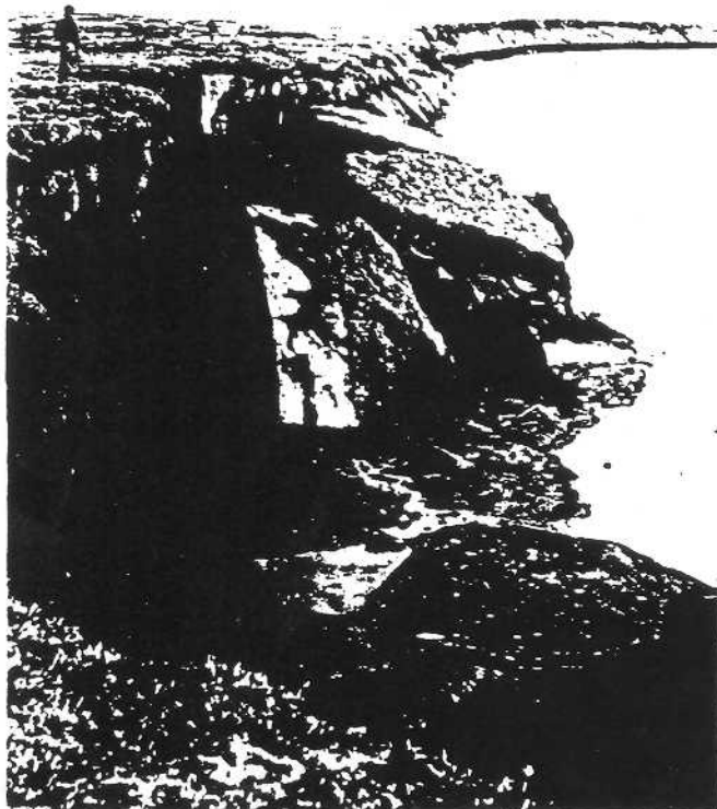
Photo 9 Collapse blocks after undercutting at Nuiqsut.
